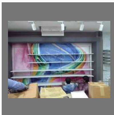
Shop Electrical Maintenance Service
