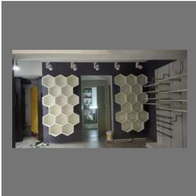
White LED Electrical Services
