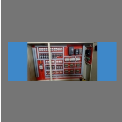
EOT Cranes Control Panel
