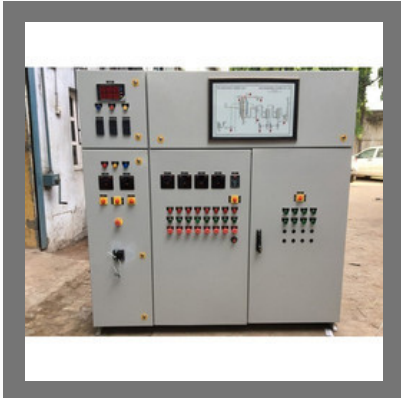
Motor Control Panel
