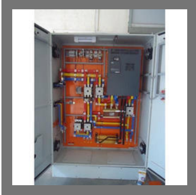
VFD Control Panel
