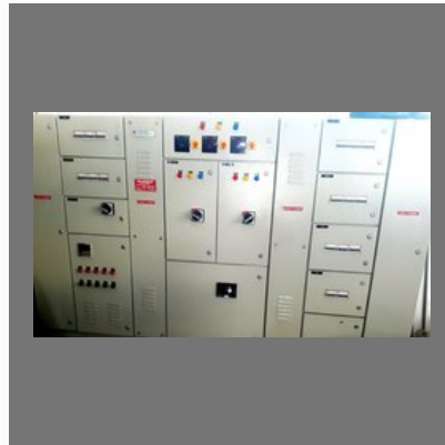
Main LT Control Panel
