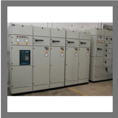
RTPFC Control Panel
