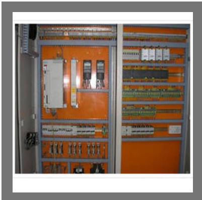
Automation Drive Panels
