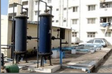
Wastewater Treatment Plant
