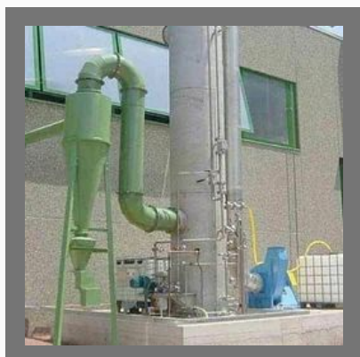
Venturi Wet Scrubber
