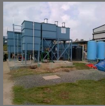
Effluent Water Treatment Plant
