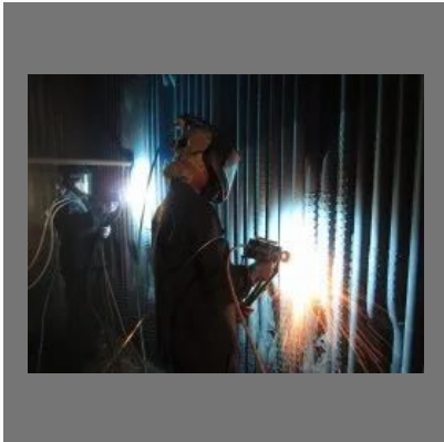
CFBC Coating On Boiler Tube
