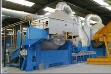
Tilting Rotary Furnace
