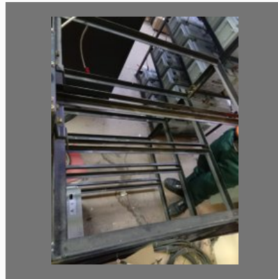
Ups Battery Steel Stand
