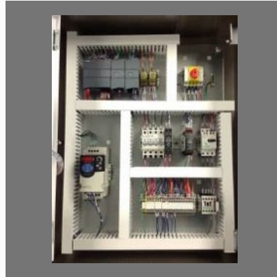
Electrical Control Panel
