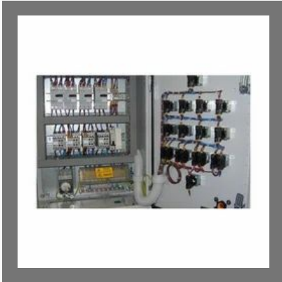
Motor Control Panel
