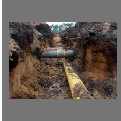
Sewer Line Facility
