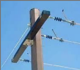
Electricity Pole Facility
