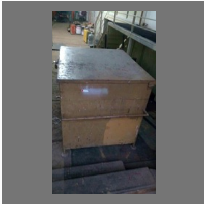
MS Oil Tanks
