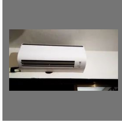
White Split Air Conditioner
