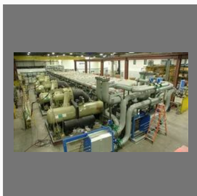
Chiller Water Treatment
