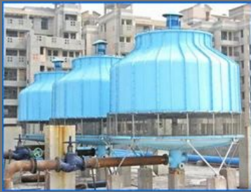
Cooling Tower Water Treatment Chemical
