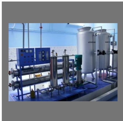
RO Water Treatment Plants
