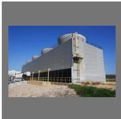
New Cooling Tower Plant & Spares
