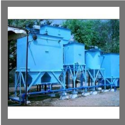
Industrial Effluent Water Treatment Plants
