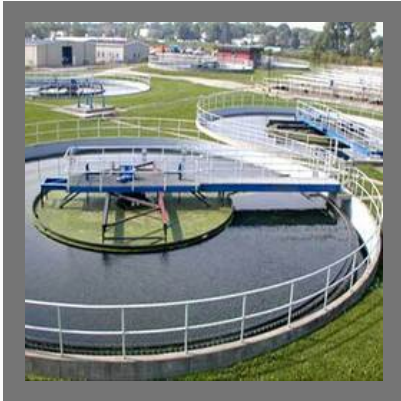
Effluent Treatment Plants
