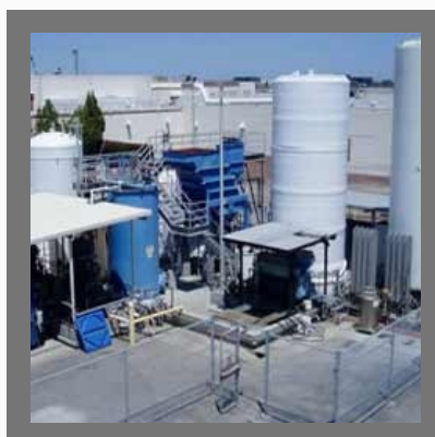
Wastewater Treatment Equipment
