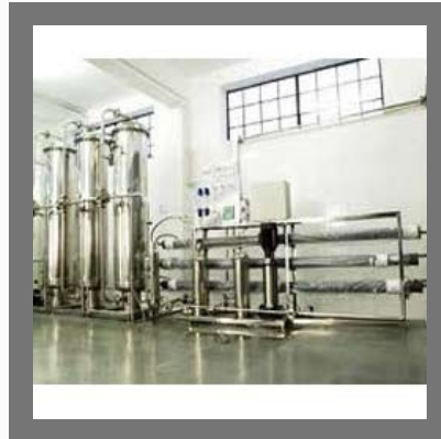
Industrial Reverse Osmosis Plants
