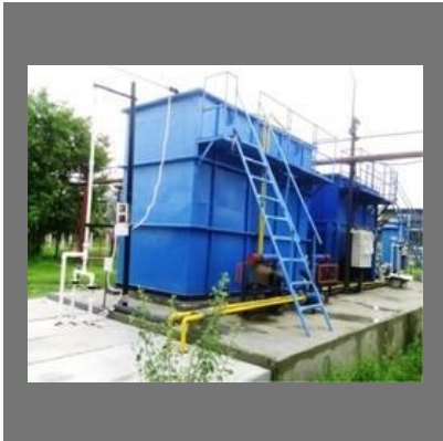
Industrial Sewage Treatment Plant
