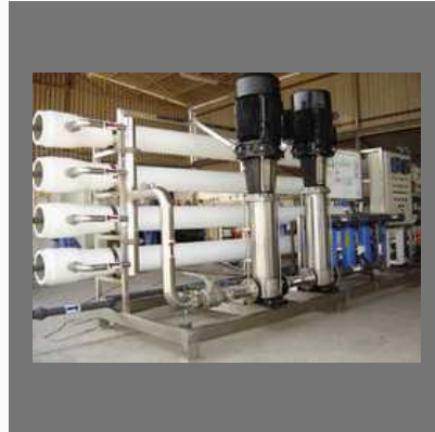
Institutional Reverse Osmosis Plants
