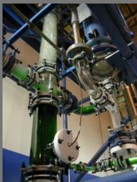
Hydrochloric Acid Recovery Plant
