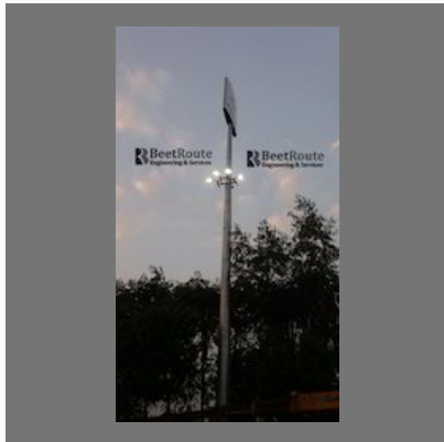
High Mast Signage With Lighting
