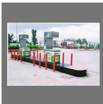
Permanently Fitted LPG Fuel Tank
