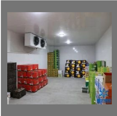
Cold Storage Chamber
