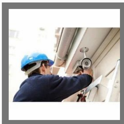
CCTV Camera Installation Service
