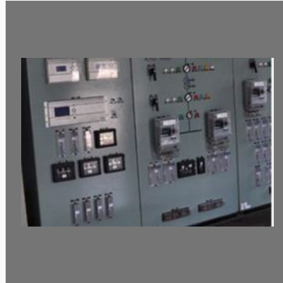
Electrical Control Panel
