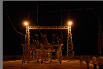
Lighting & Earthing Systems
