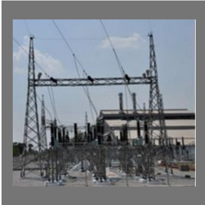
EHV Transmission lines
