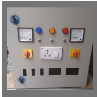
Electric Control Panel
