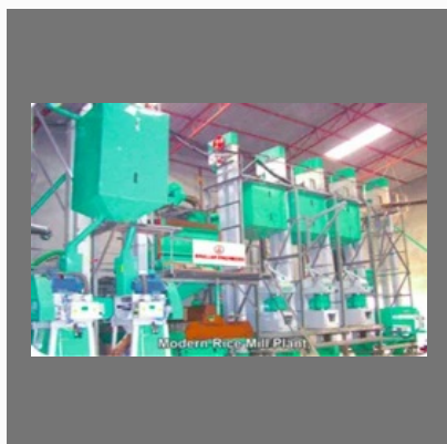
Rice Mill Plant
