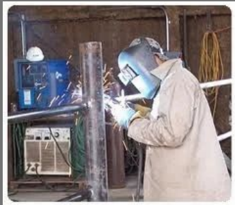
Mechanical Works Service
