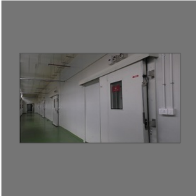
Cold Room Storage
