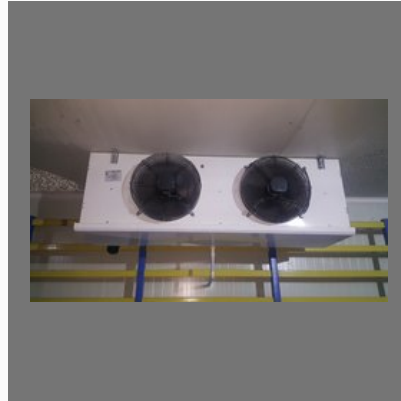
Pharmaceutical Storage Cold Room
