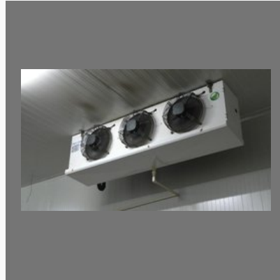
Dairy Cold Rooms & Storage
