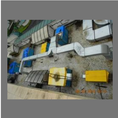
HVAC Ducting System
