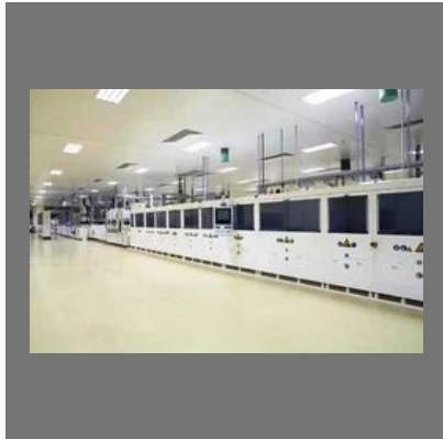
Clean Room Equipment
