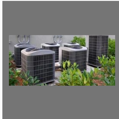
VRF Air Conditioning System
