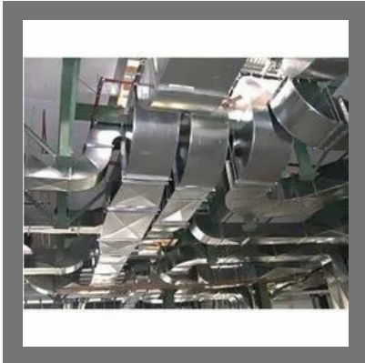
Annual Maintenance Contract For HVAC Systems
