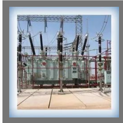
Electrical & BMS Project Services
