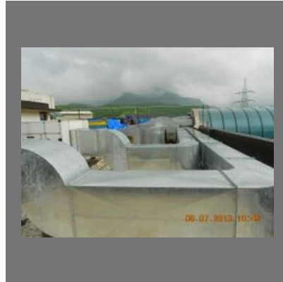
HVAC Ducting Service
