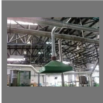
MS Air Duct
