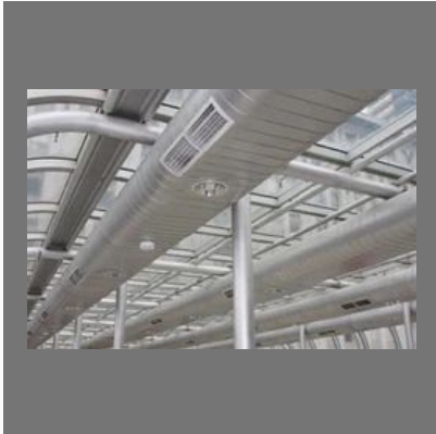
Air Conditioning Duct
