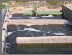
Effluent Treatment Plant
