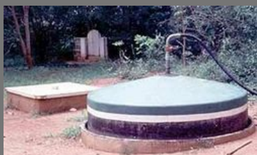
Bio Gas Energy Generation
