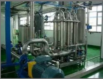
Laundry Waste Water Treatment
