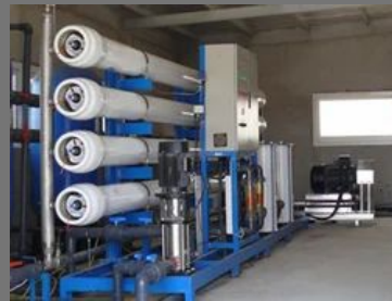
Desalination By Reverse Osmosis Plants
