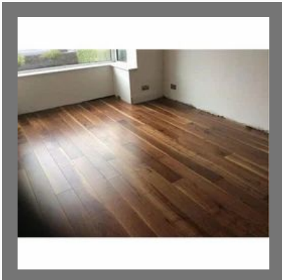
Laminated Wooden Flooring
