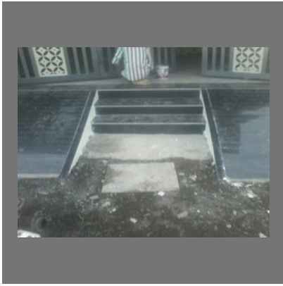
Granite Fitting Services
