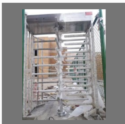
Access Control Turnstile
