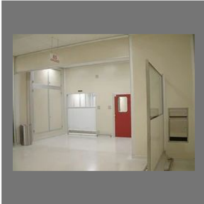
Clean Room Wall Panel
