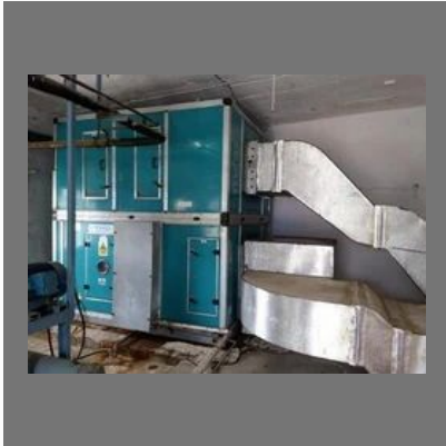
AHU Duct Service
