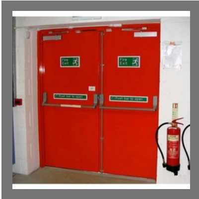
Push Bar Fire Exit Door
