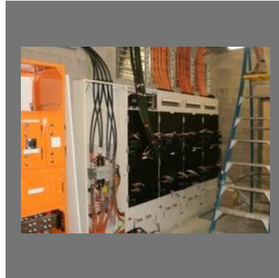
Commercial Electrical Works
