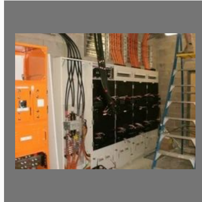
Commercial Electrical Works
