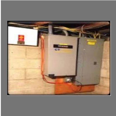
3 Phase Electrical Service
