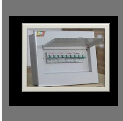
Interior Electrical Services
