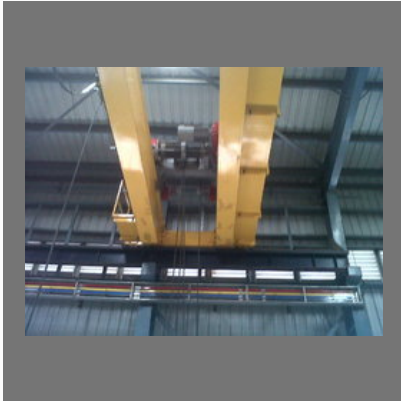
Double Girder Cranes
