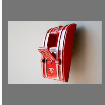
Patriots Hotel Fire Alarm
