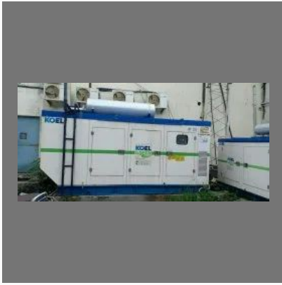
Kirloskar Diesel Generator 250kva
