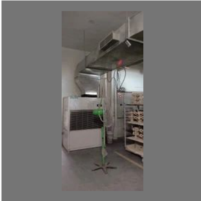
Industrial Ac Duct
