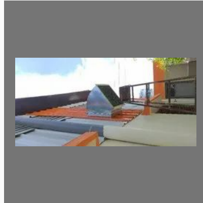
Compressor Air Duct
