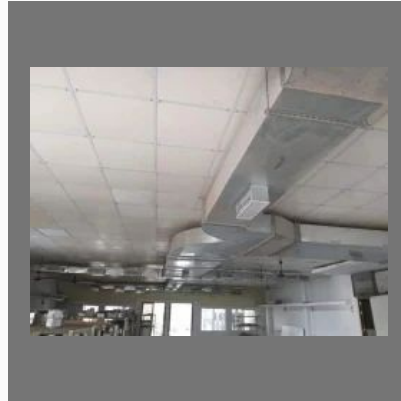
HVAC Ducting System
