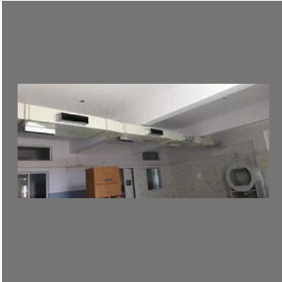
Air Conditioning Ducting Service
