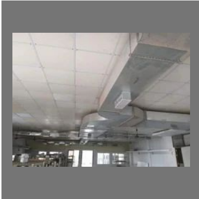
Central Air Conditioning System
