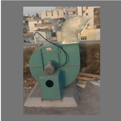
Air Exhaust Blower
