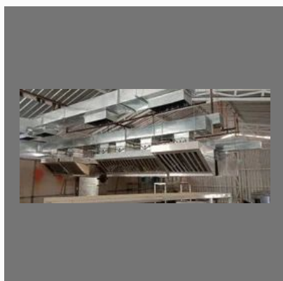
Hotel Ss202 Commercial Kitchen Chimney
