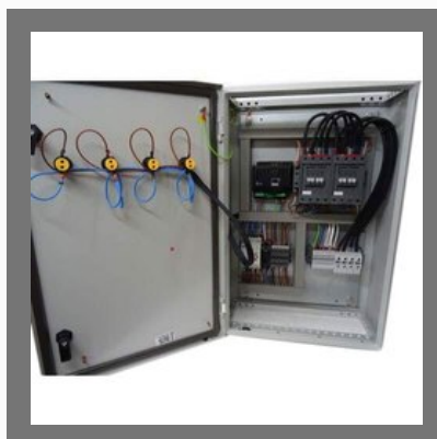
LT Distribution Panel
