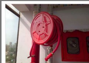
FIRE HOSE REEL
