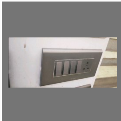
Electrical Switch Board
