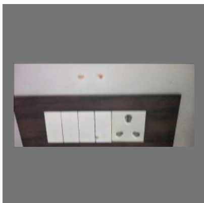
Electrical Switch Board
