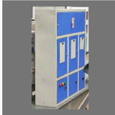
Control Panel Box
