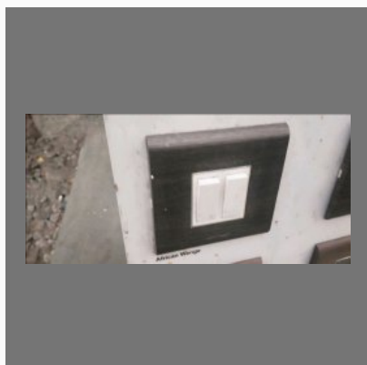
Electrical Switch Board
