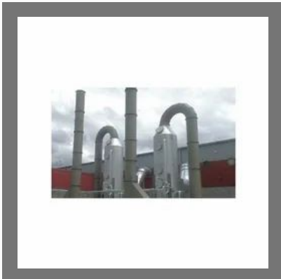
Industrial Scrubber System
