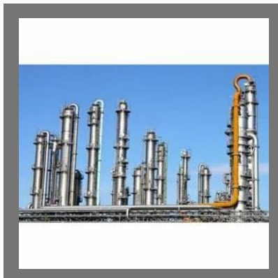
Industrial Distillation Plant
