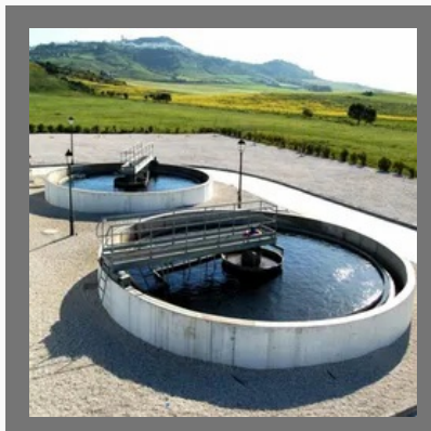
Effluent Treatment & Wastewater Treatment Plant
