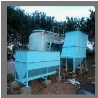
ETP Effluent Treatment Plant
