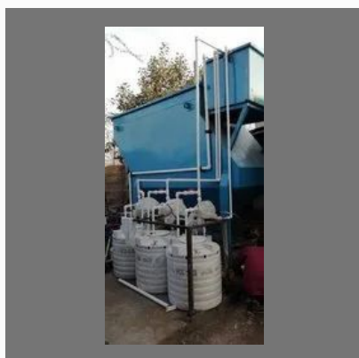
dairy effluent treatment plant
