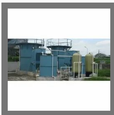
Effluent Treatment Plant
