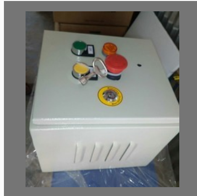
Siemens Drive Panel
