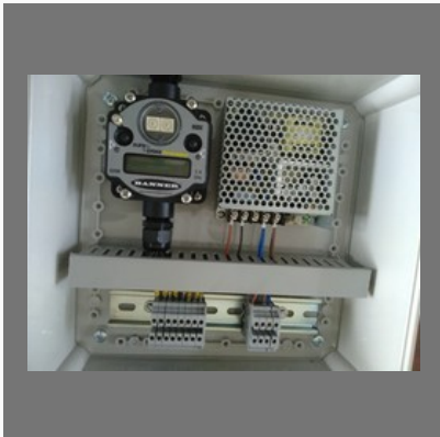
Wireless Control Panel
