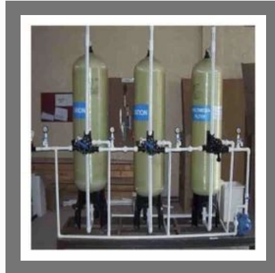
Dm Water Plant
