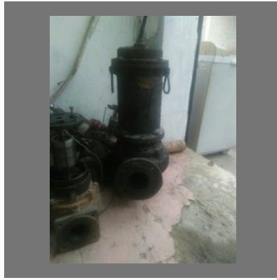
Sum Pump Rewinding
