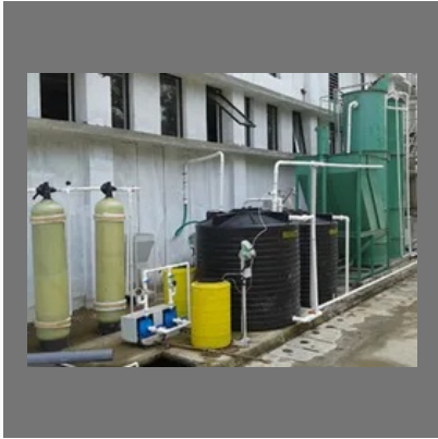
Sewage Treatment Plant
