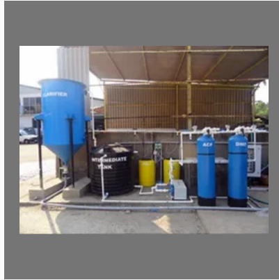
Effluent Treatment Plant
