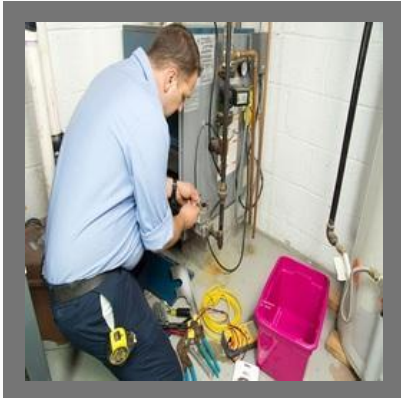
Air Conditioning Contractor
