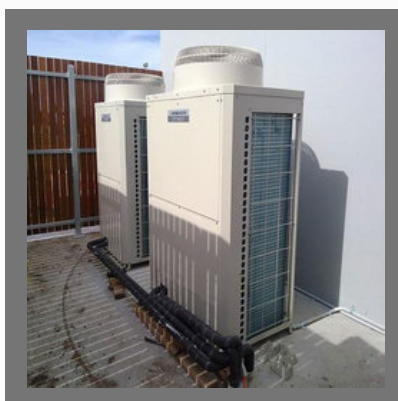
VRF Maintenance Service
