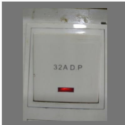
Anchor Main Switches
