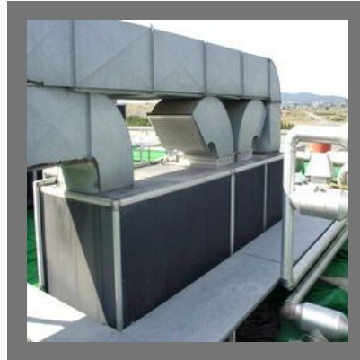
Air Conditioning Plant
