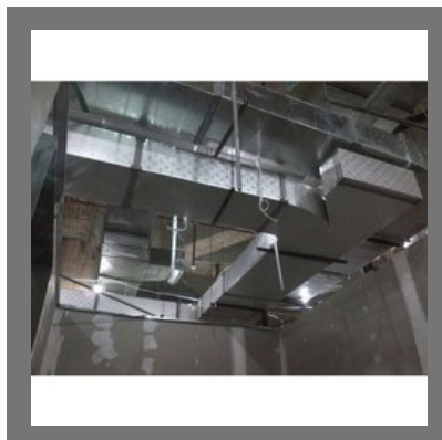
GI Ducting For HVAC System
