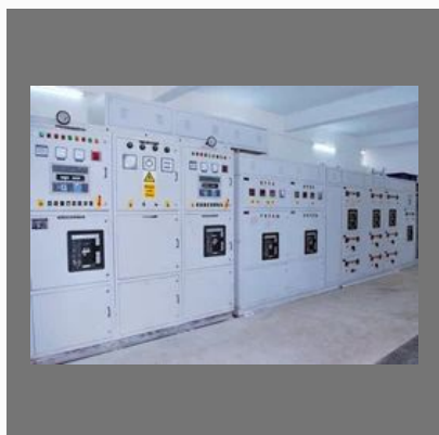
Breaker Panels & Acb Panels
