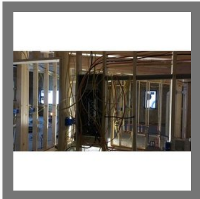
House Wiring Service
