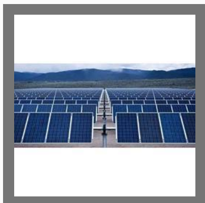
Solar Power Plant
