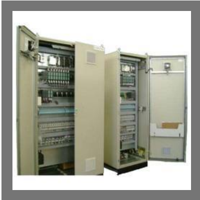
PLC Based Control Panel
