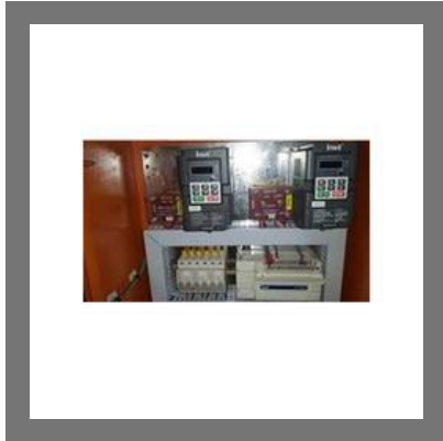
Variable Speed Drive Panel
